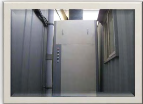
AIR CONDITIONING EQUIPMENT
