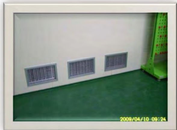
AIR CONDITIONING EQUIPMENT
