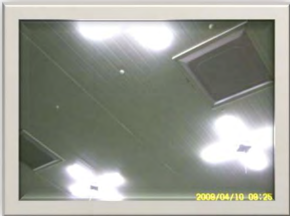
AIR CONDITIONING EQUIPMENT
